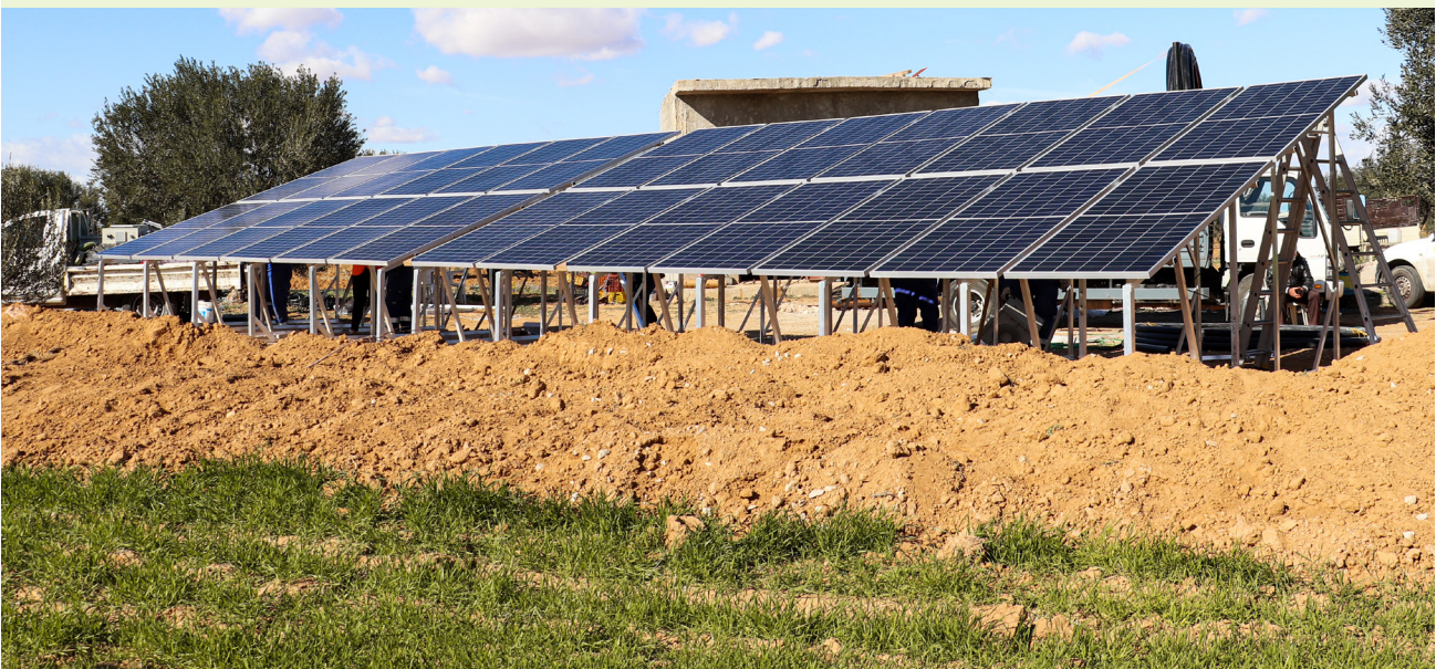
Figure 3. 10.4-kWp solar PV water pumping system for farm of Abdallah Ben Mansour in Chorbane
